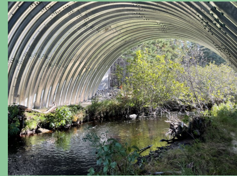
An example of a recently installed large arched culvert over a brook showing the maintenance of the brook's natural flow.
